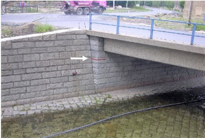
Fig. 6 Flood warning marker on the Müglitz (Picture: Paus)
